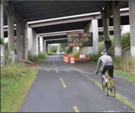
The W&OD trail is temporarily shifted under the Dulles Toll Road (Route 267). Photo by Trevor Wrayton, VDOT
