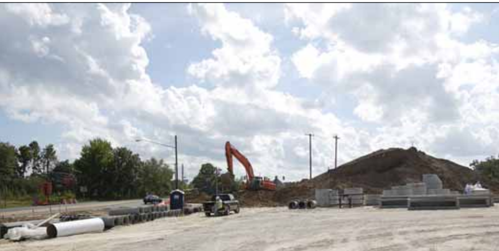
Park & Ride Lot expansion is underway in Prince William County at Route 234. Photo by Trevor Wrayton, VDOT
