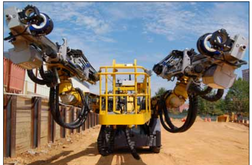
At the Dulles Metrorail project, crews rely on the "Drill Jumbo" to tunnel from Rt. 123 to Rt. 7. Photo courtesy Dulles Transit Partners
